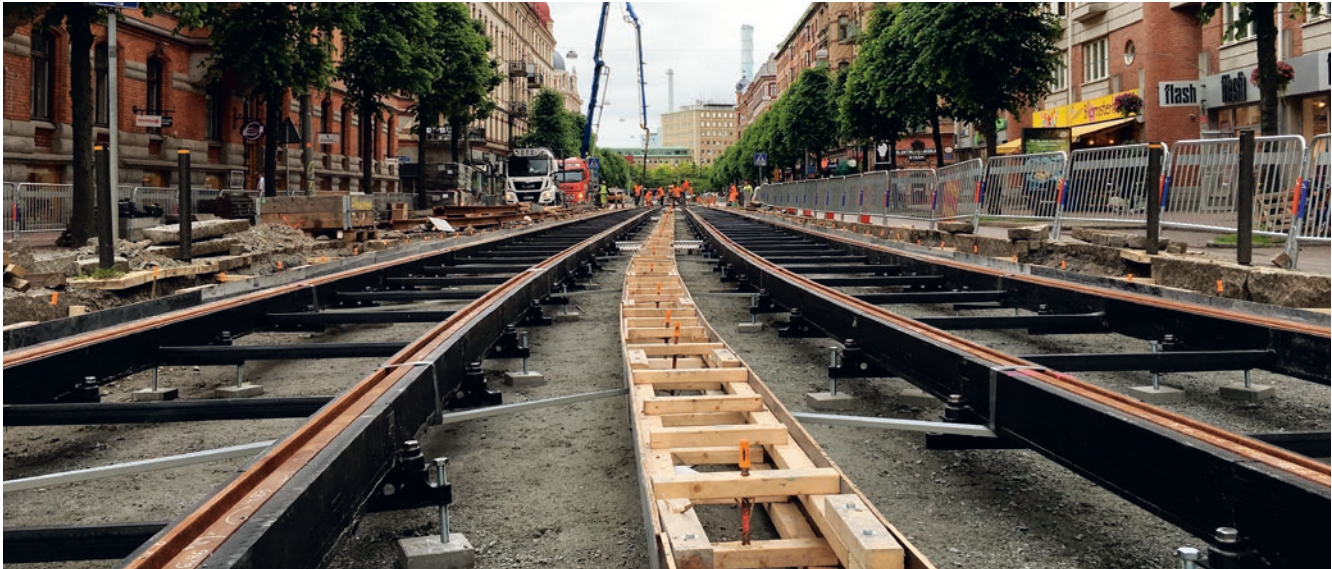
To reduce leakage current and vibrations, girder blocks and green rails were installed in Mölndal and Gothenburg.
